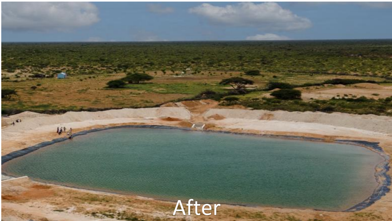
The Newly constructed Haffir dam in Kalluun-Dacar village in June 2024 (Photo Credit/Galmudug PIU).
